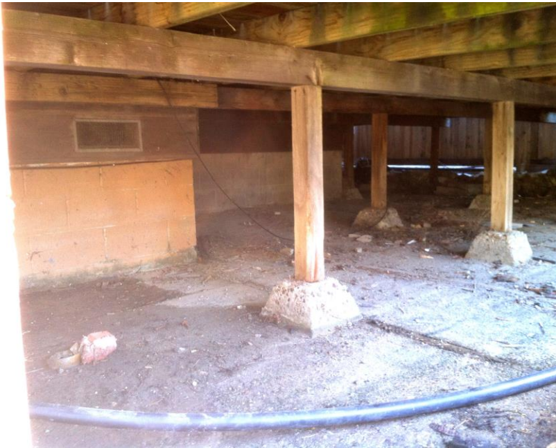
Stem wall foundation & deck piers (from rear). All flood openings are more than 1.0' above adjacent grade.
